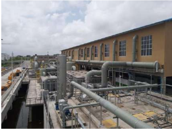
Leachate Treatment Plant and Deodorization System
